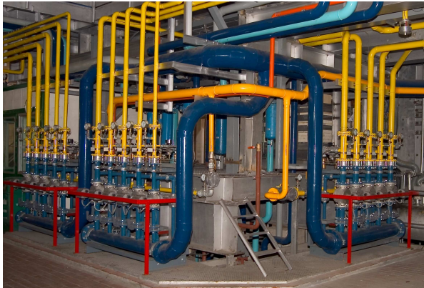
Figure 2 - 3 SORG air/gas control stations featuring the VMC system
