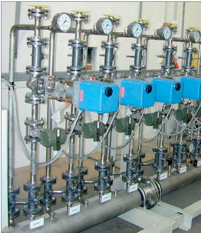
Oxygen station for individual burner control
