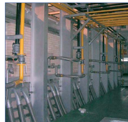
Burner installation on a SORG® oxy-fuel furnace
